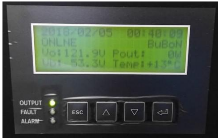
1. Red Alarm – LED FLASHING
