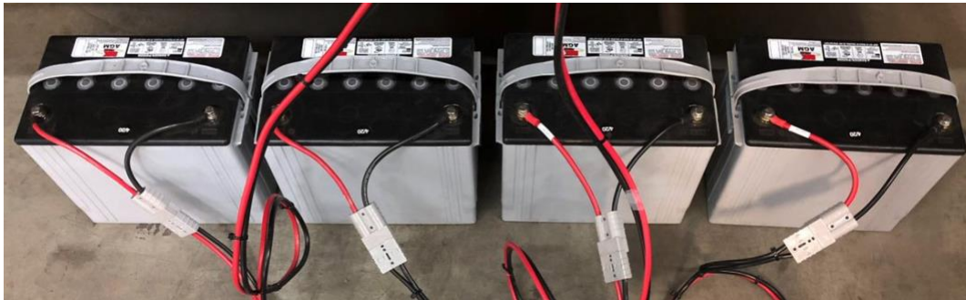
BATTERIES CONNECTED TO BATTERY HARNESS
