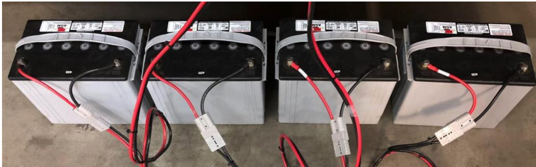
BATTERIES CONNECTED TO BATTERY HARNESS
