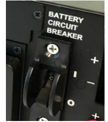
BATTERY CIRCUIT BREAKER
