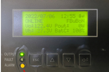
1. Yellow Alarm LED ON
