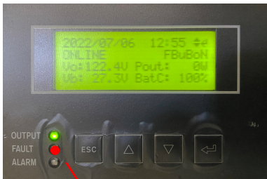
1. Red Fault LED on
