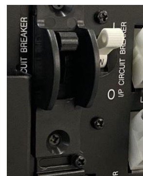
BATTERY CIRCUIT BREAKER
