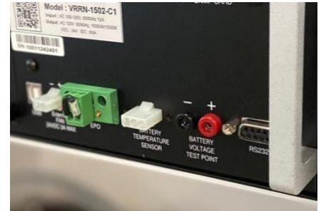
BATTERY TEMPERATURE SENSOR
